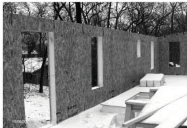
A construction photo shows the eight-inch-thick wall insulated with foam, sandwiched between two layers of particle board.
